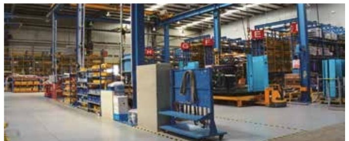
Oil injected screw compressors and Refrigerated Dryer plant: Pan-Asia, Wuxi
